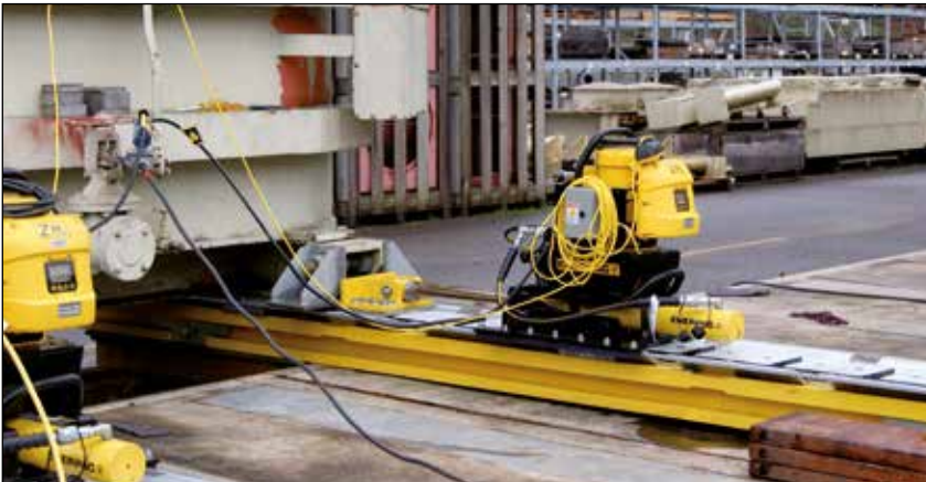
▼ A custom hydraulic Low-Height Skidding System will provide the maintenance team with the ability to maneuver and transport transformers with physical access limitations.
